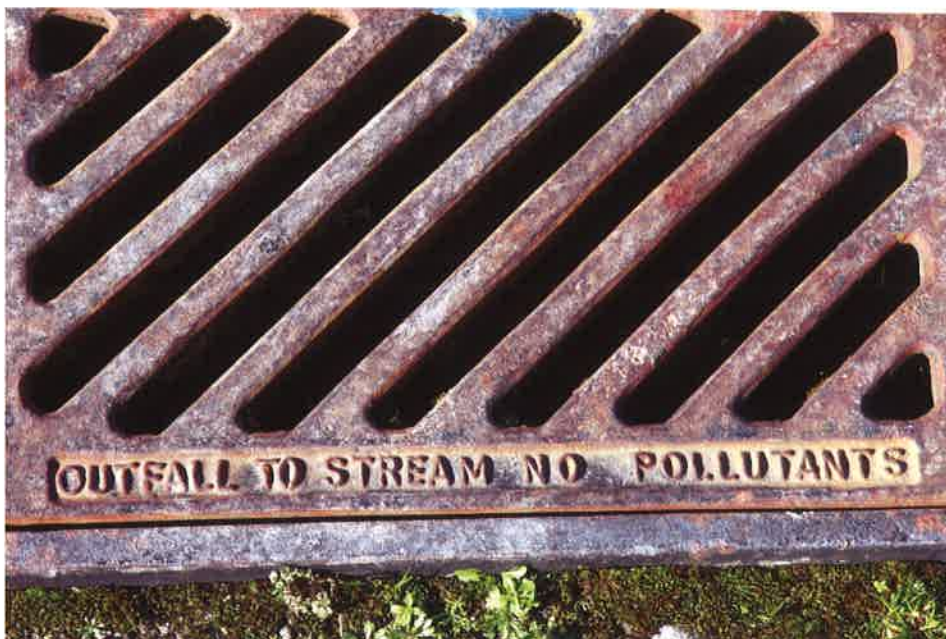
Any polluted water that flows through this drain goes directly to a stream.
